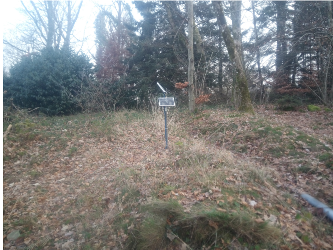
Figure 3.2: Solar panel configuration
